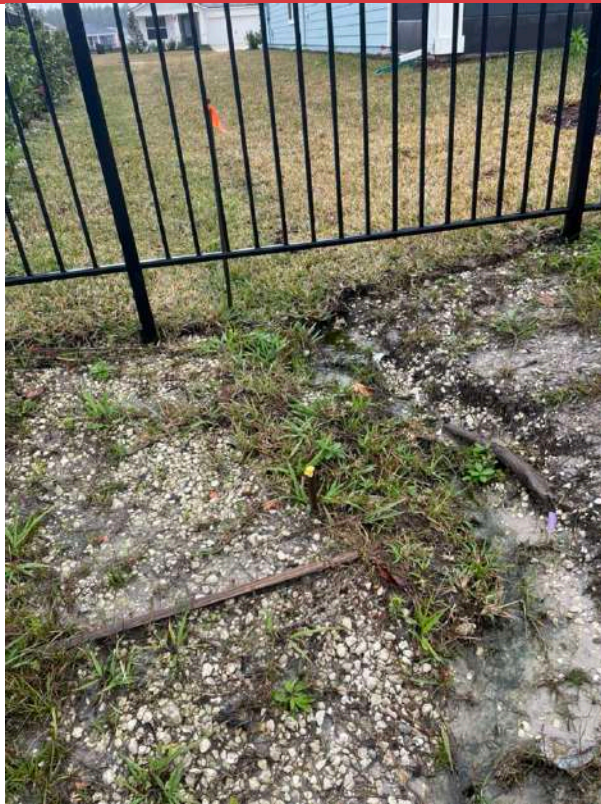
WASHOUT BEHIND HOMES
