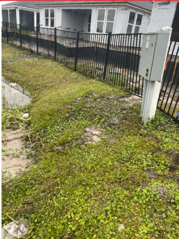
UNEVEN POND BANK Cannot get mowers past corner
